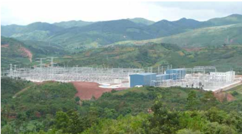
Fig. 3: UHV DC Sending Station Chuxiong in Yunnan, China
