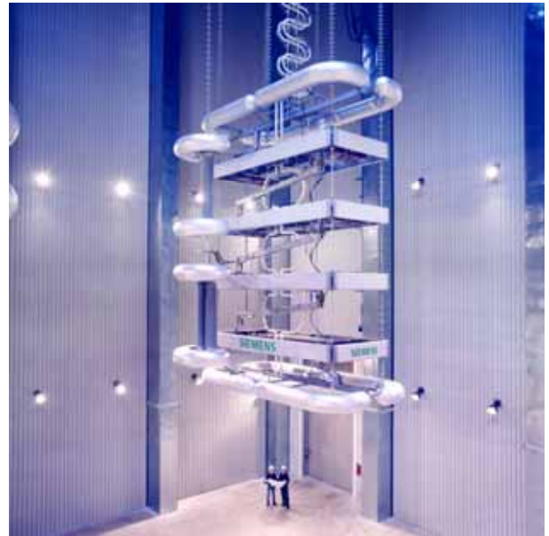
Fig. 2: UHV DC Valve Tower in the Cologne testing laboratories
