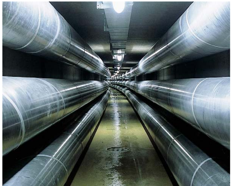
Fig. 3: Tunnel laid GIL as operation at the Geneva Airport since 2000
