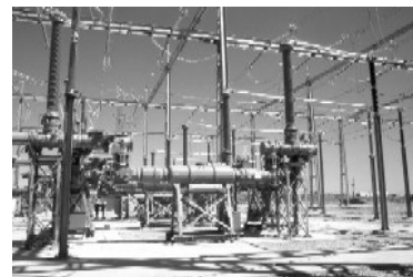
Fig 7: HIS installation in Spain (400 kV, commissioned 2005)
