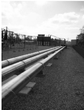
Fig 9: GIL connecting HIS and GIS in outdoor installation
