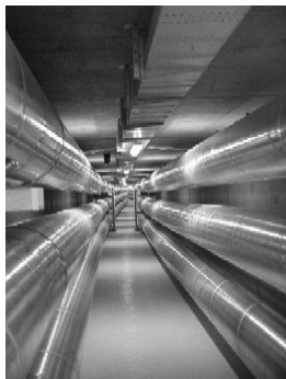
Fig 4a: Tunnel installed GIL in Geneva
